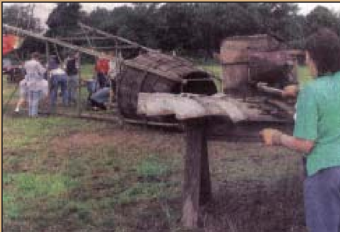
Board members and volunteers of the Northern Neck Farm clean and restore a donated windmill.
